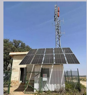
Green off-grid site. Image property of Cellnex.
